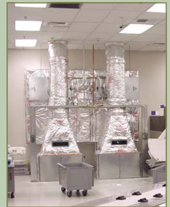
Interior Paper Collecting System
